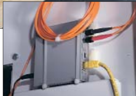
Fiber optic cable
